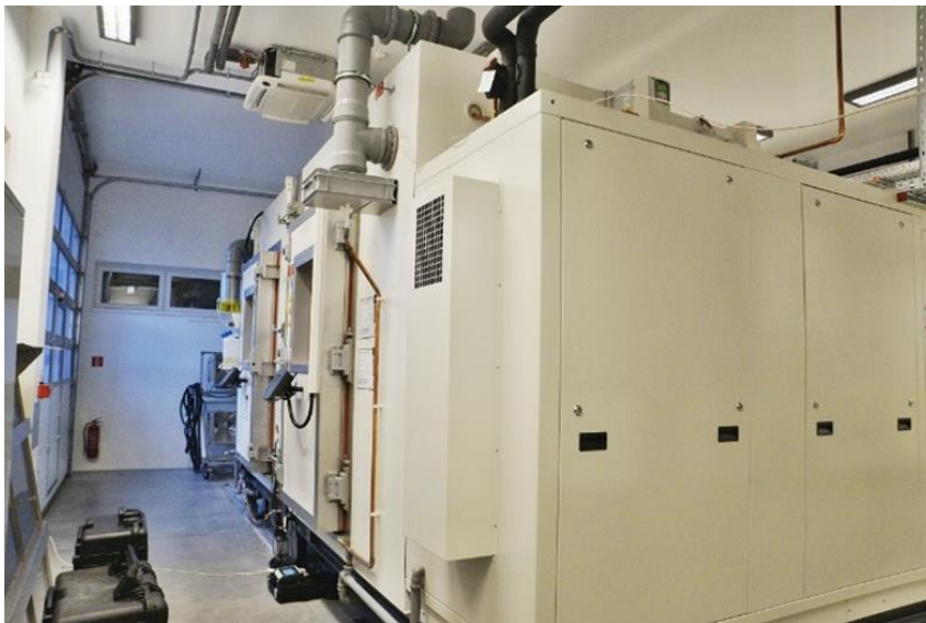
Fig. 2 View of the climate chamber of Department of Building Engineering and Urban Planning
